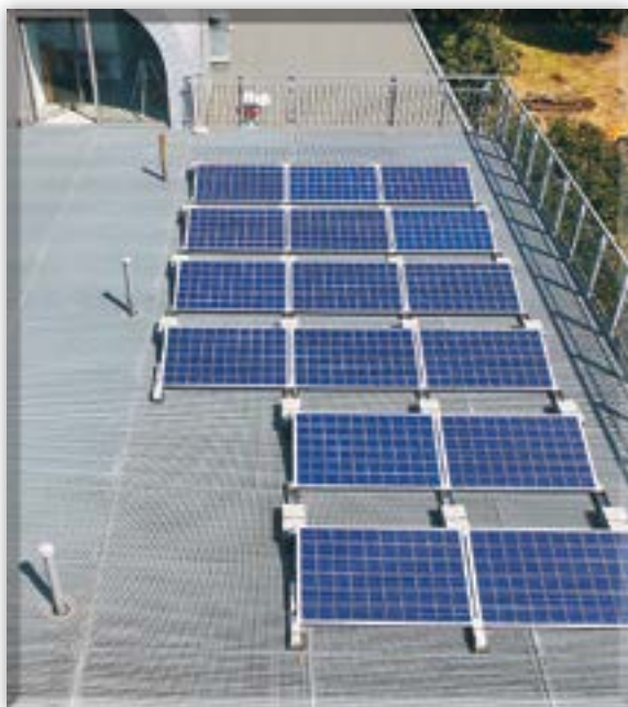
Solary na dachu
